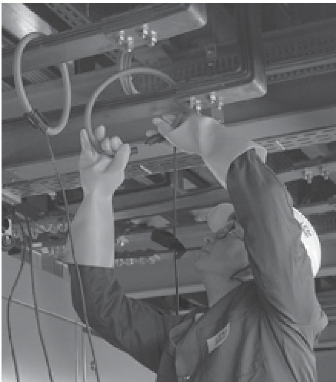
Fig. 40 Typical LEM-flex use, surrounding conductor(s) and latched.
